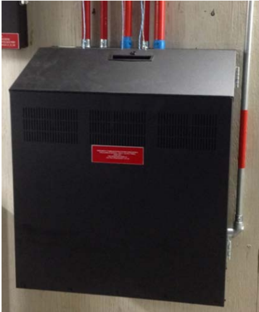
Figure 4-10: Fire Alarm/Textual ECS Interface Cabinet
