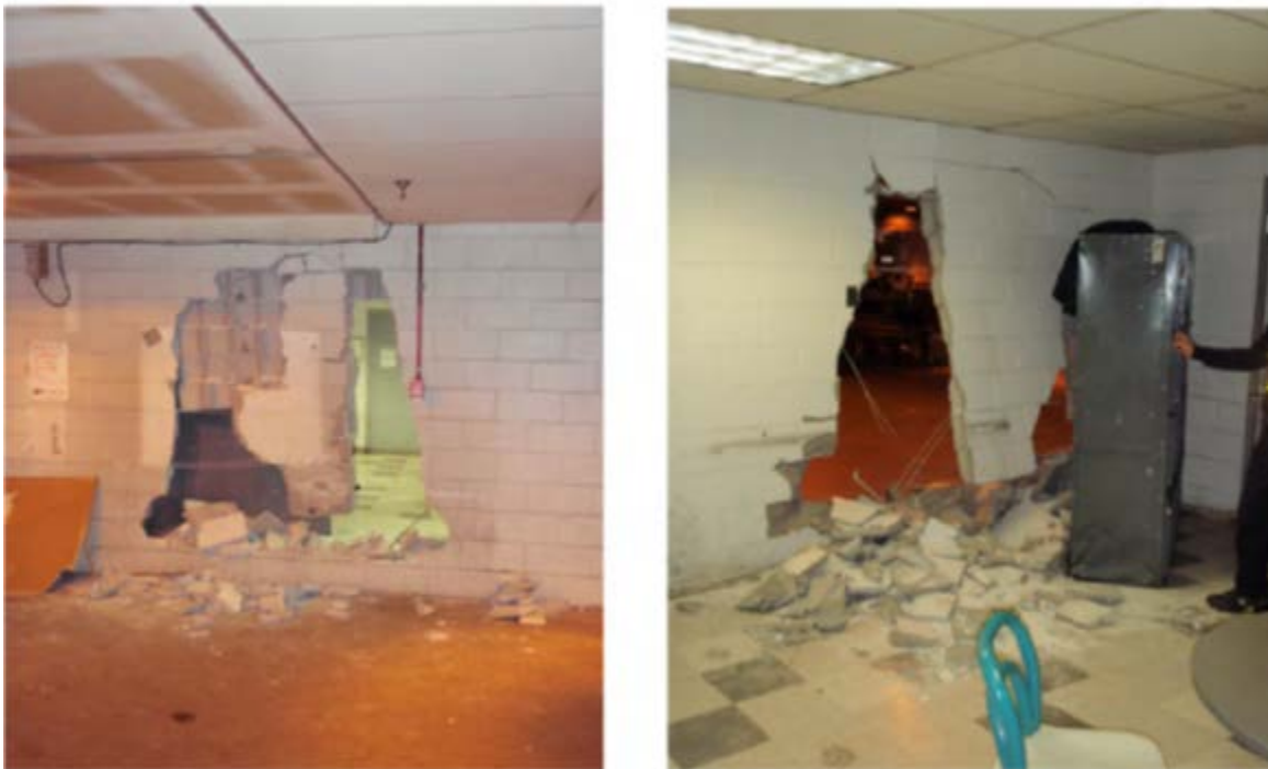
Figure 5.8-1: Concourse B: Tug Damage to Wall
