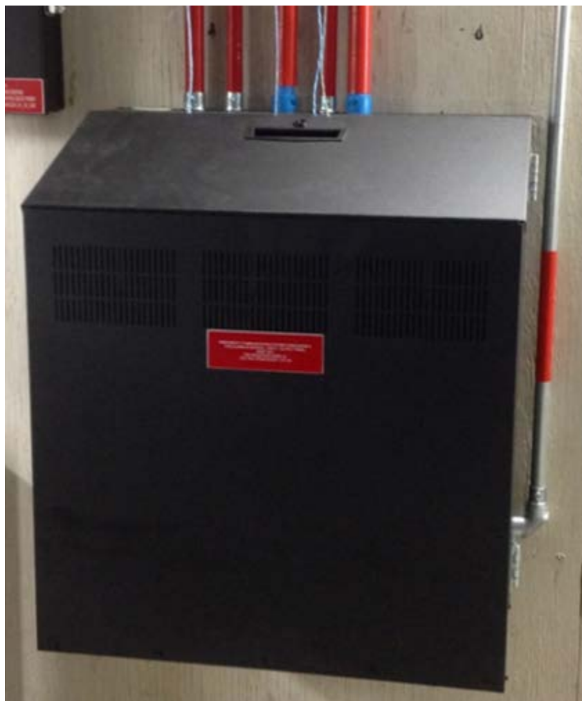
Figure 4.4-6: Fire Alarm/Textual ECS Interface Cabinet
