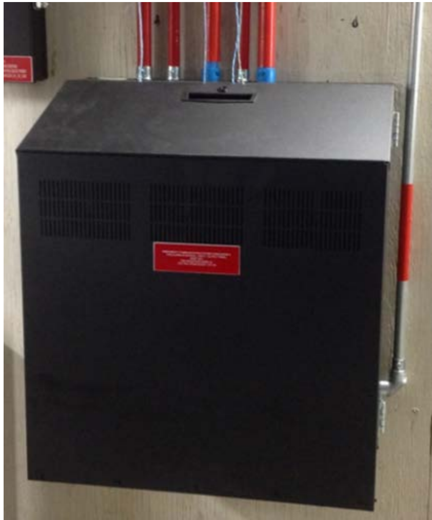
Figure 4-6: Fire Alarm/Textual ECS Interface Cabinet
