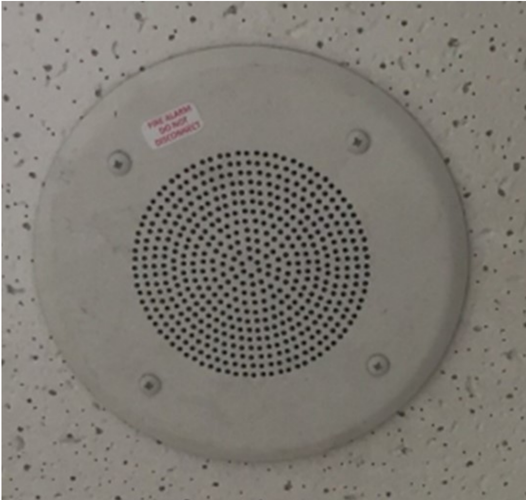
Figure 4-1: Typical Ceiling Loudspeaker with ECS Indicator
