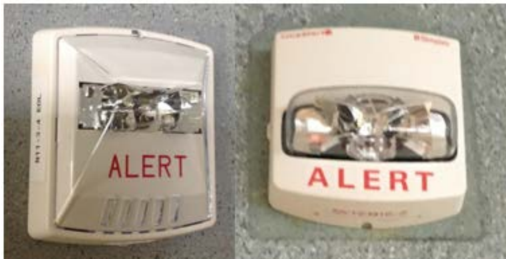
Figure 4.3-1: Typical ALERT Strobes
