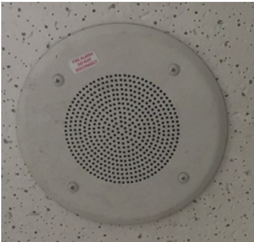
Figure 4.4-1: Typical Ceiling Loudspeaker with ECS Indicator
