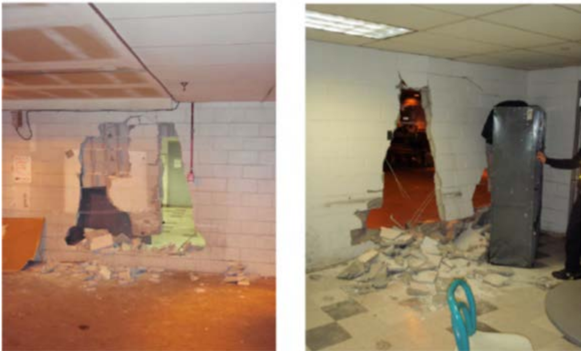
Figure 5.8-1: Concourse B: Tug Damage to Wall
