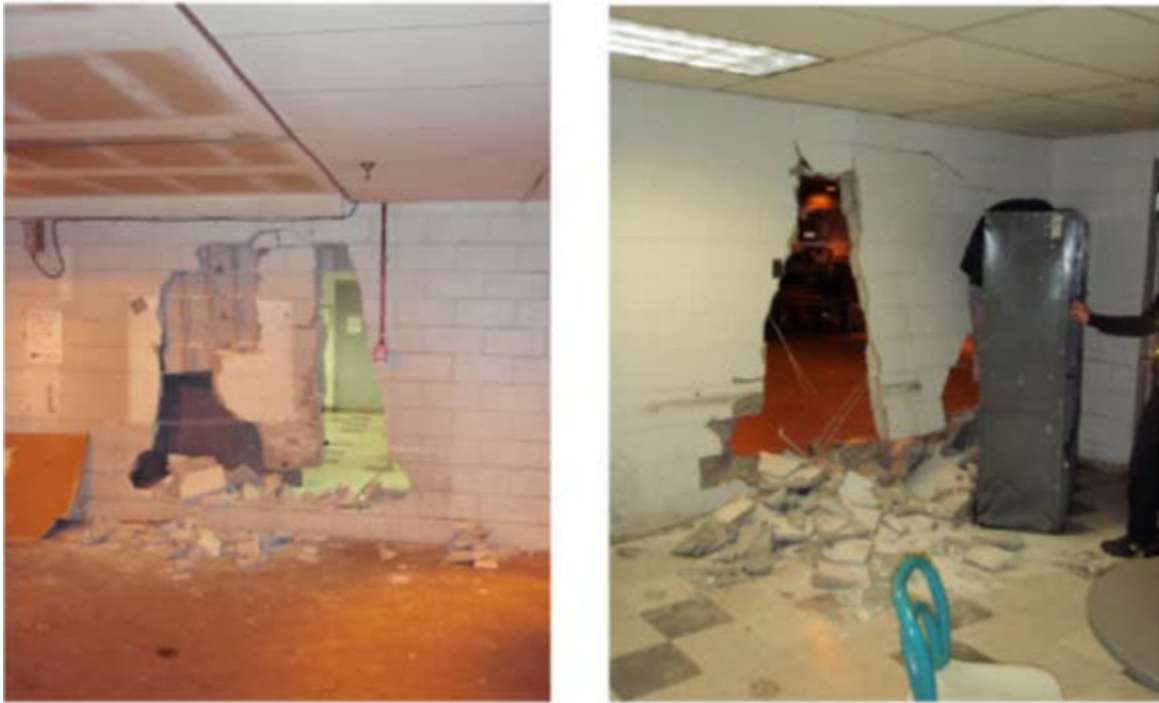
Figure 8-1: Concourse B: Tug Damage to Wall
