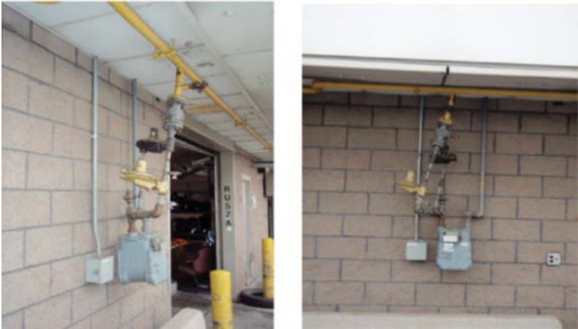
Figure 8-2: Gas Piping Strike: Side and Front Views
