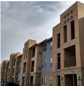
Fiber cement panels unexceptionable.
